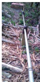
Self Installed Supply Pipe
