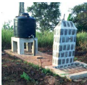
Storage Tank and Tap
